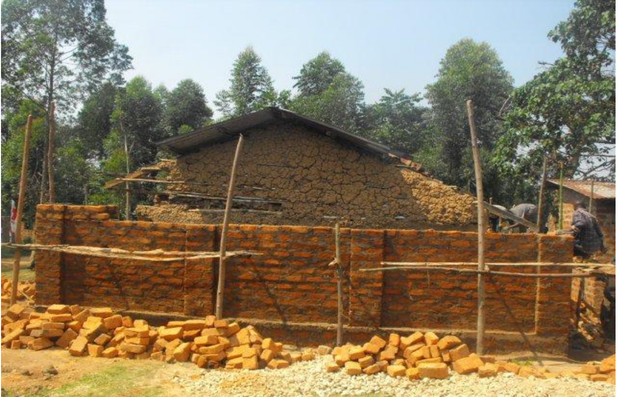
Mercy Children's Academy at the start of the construction in August of 2010.
